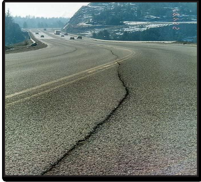
Figure 4: Typical Longitudinal Cracking (12)
