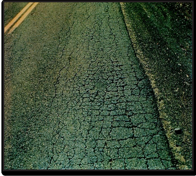
Figure 2: Typical Fatigue Cracking (12)
