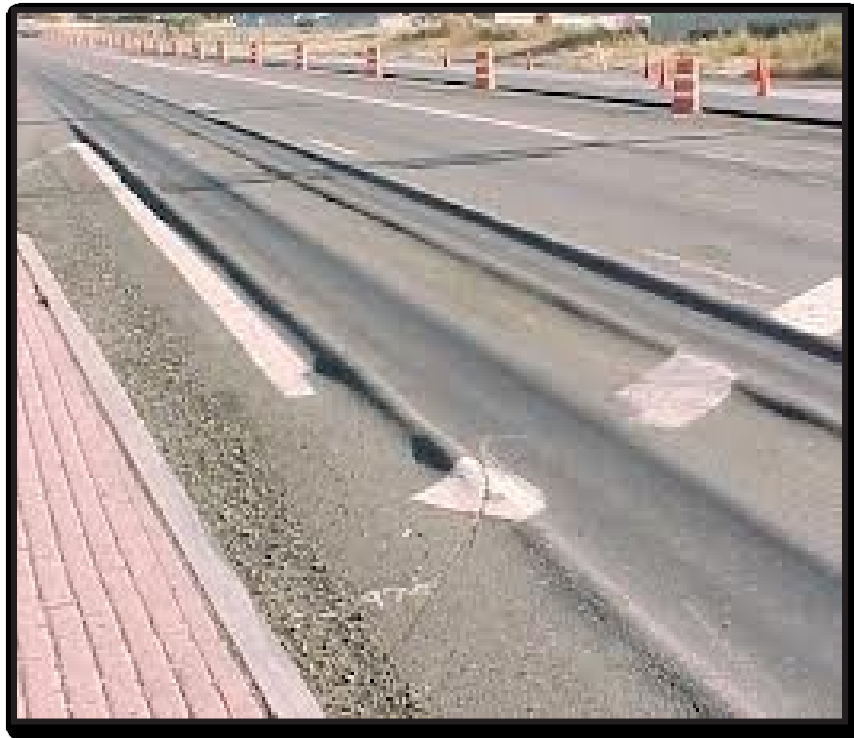
Figure 1: Typical Rut in a Flexible Pavement (12)
