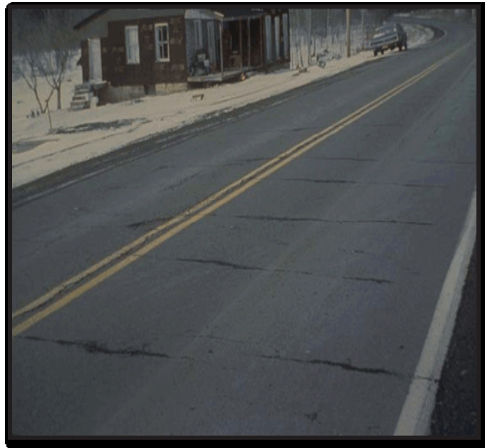
Figure 3: Typical Transverse Cracking (14)
